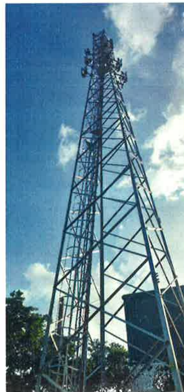
Bangalore - Roof Top Tower Tippenhalli
