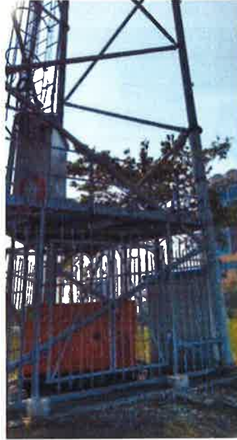
Kolkata - Ground Based Mast Rajarhat
