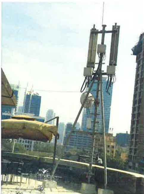
Mumbai - Roof Top Pole Reliance Jio SRM Office, Worli
