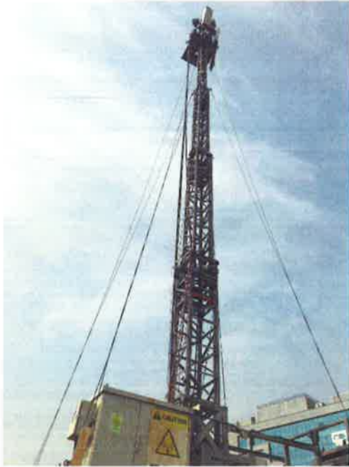
Mumbai - Cell on Wheels Bandra Kurla Complex
