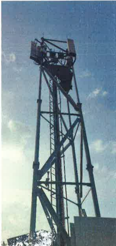
Bangalore - Roof Top Tower Rajaji Nagar
