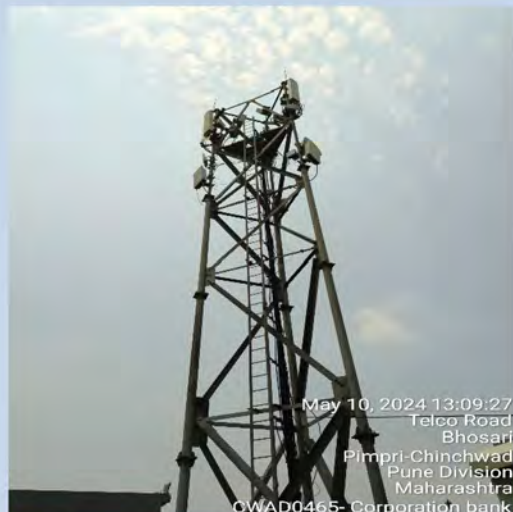
Corporation Bank, Bhosari, Pune
